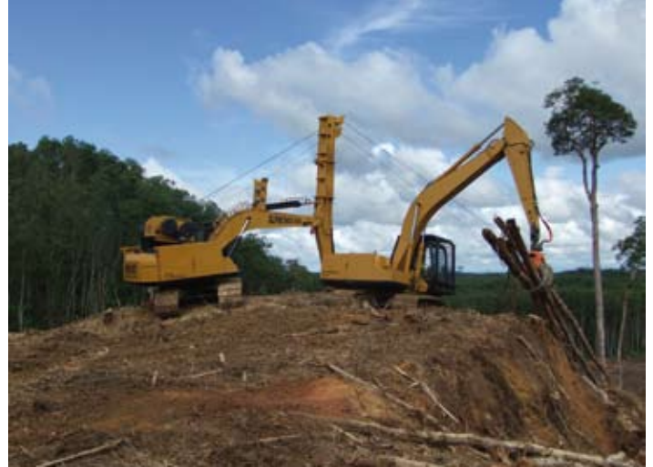
The excavator, fitted with a timber grab, was used to clear the chute in front of the high production shovel yarder.
